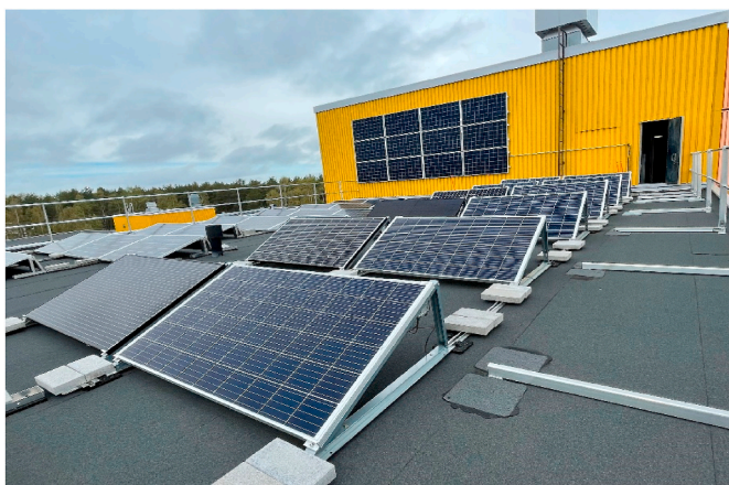
Fig. 4. The research infrastructure comprises 12 vertical solar PV panels and 12 rooftop inclined solar PV panels.
