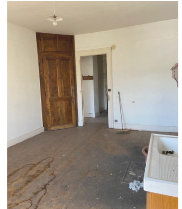
Fig.37 : The existing wooden floor is in bad condition and there is also marks of humidity damages.
