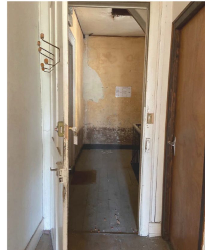
Fig.36 : The corridor giving access to the apartment. We can see the poor condition of the flooring and walls coating.
