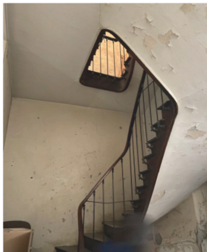
Fig.25 : The stairs to access to the ground floor from inside is not in good condition.
