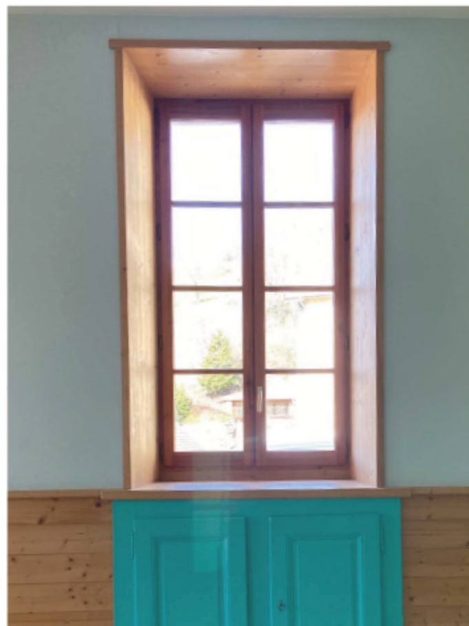
Fig.41 : We can see the thickness of the load bearing walls on the upper floors (50cm).
