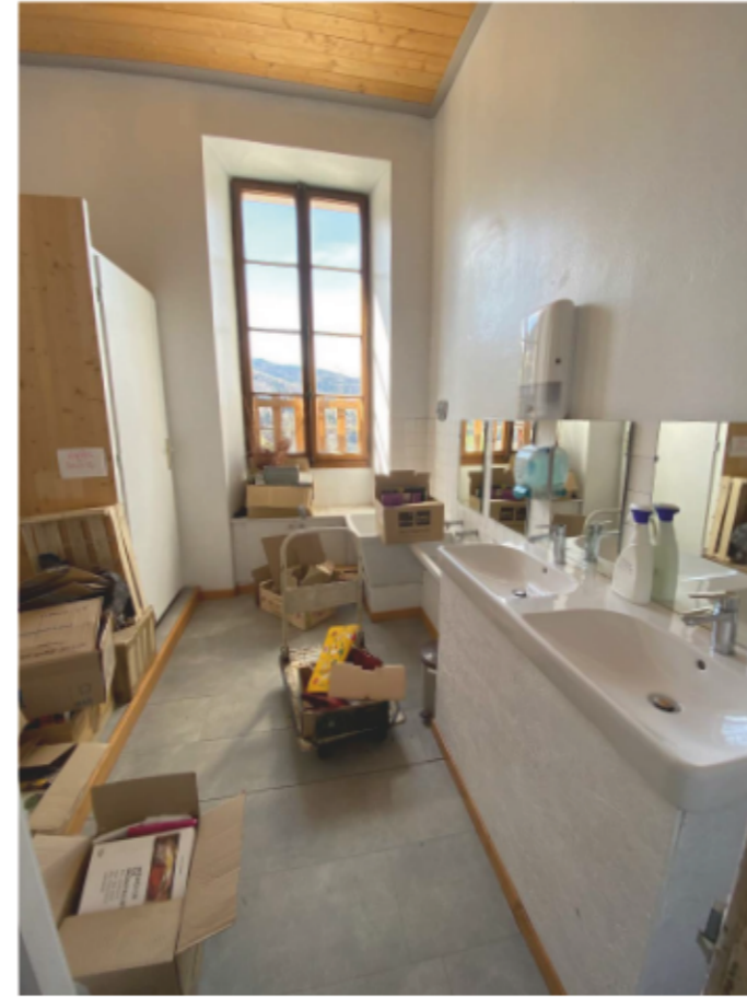
Fig.34 : The sanitary space that is also used as a storage space. I guess that it is not used anymore.
