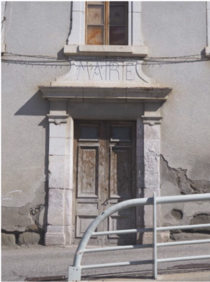
Fig.22 : The original main door with its moldings is not in used anymore because of the busy road that runs along the facade. In French «Mairie» means «City Hall». © Angèle Golliet
